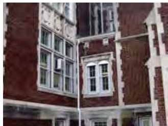
EXISTING SECURITY GRILLE Replace existing metal grille and windows with new security glazing at lower two floors, per DCPS guidelines, typical throughout.
