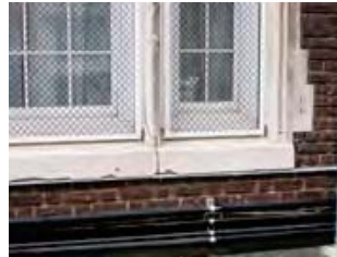
EXISTING STONE Replace damaged existing stone as required - typical throughout
