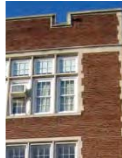
EXISTING WINDOWS Replace existing windows with new low-E windows per DCPS guidelines, typical throughout.
