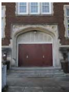
EXISTING EXTERIOR DOORS Replace existing metal doors with new paneled doors per DCPS guidelines and historic photographs, typical throughout.
