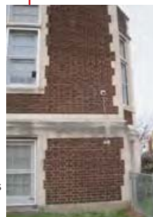
SECURITY Replace security cameras and conceal conduit - typical throughout
