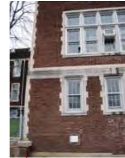
EXISTING MASONRY Clean and repoint stone and bricks as required - typical throughout
