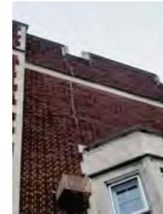
MASONRY CRACK Repair cracked brick at exterior wall.
