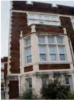
EXISTING MASONRY Clean and repoint stone and brick as required - typical throughout
