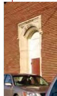
EXISTING EXTERIOR DOORS Replace existing metal doors with new paneled doors per DCPS guidelines and historic photographs, typical throughout.
